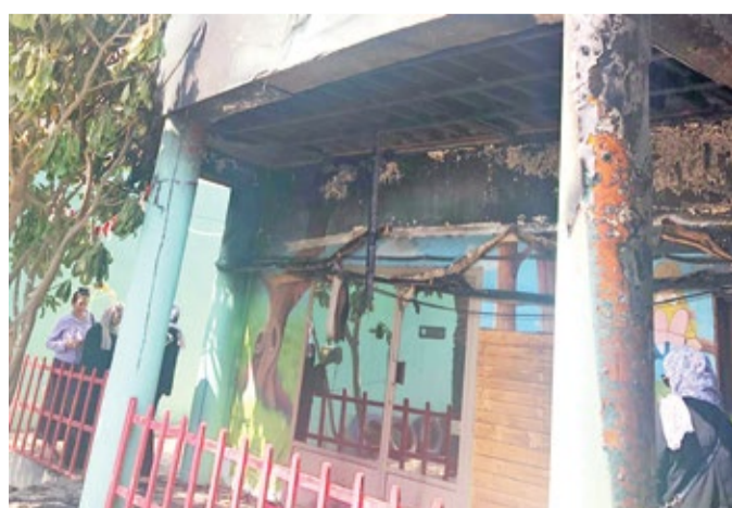
A portion of the kindergarden was damaged in the fire.
